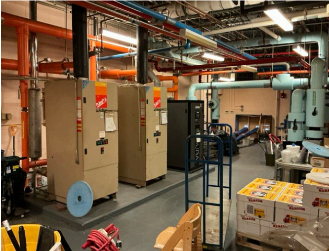
25 - MAIN MECHANICAL ROOM
