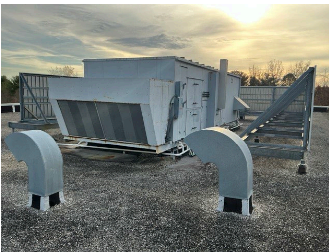
35 - ROOFTOP MECHANICAL EQUIPMENT
