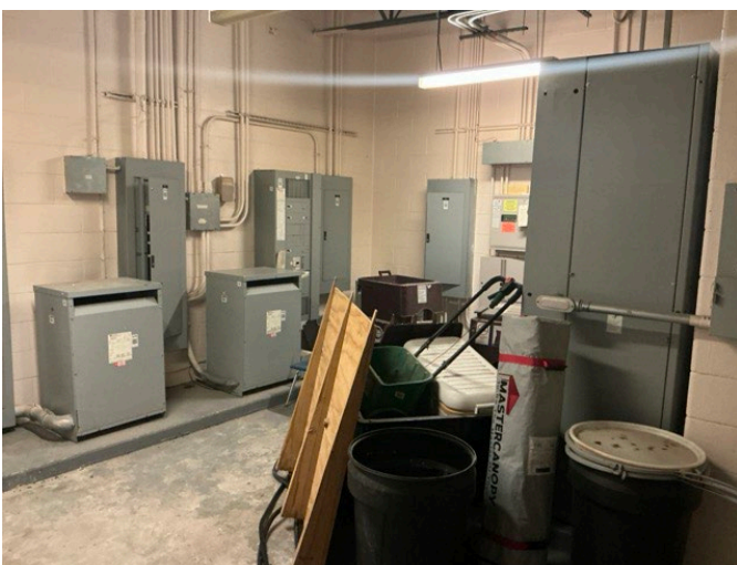
29 - MAIN ELECTRICAL ROOM
