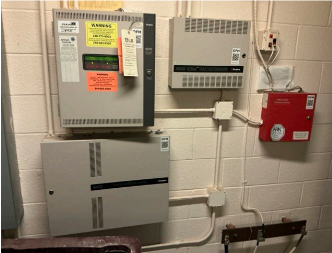
31 - FIRE ALARM PANEL
